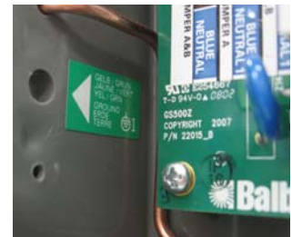
Ground in System Enclosure
